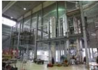
EoN Karlshamn Sweden - 5 MWth Chilled Ammonia - Fuel
